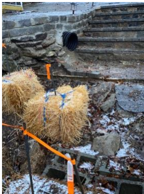
Dobush Right of Way – No 'First Flush' Discharge Non-Functional Drain
