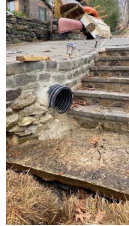
Dobush Right of Way – No 'First Flush' Discharge
