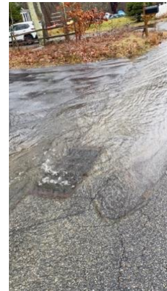
Erdoni Road Culvert Overflow
