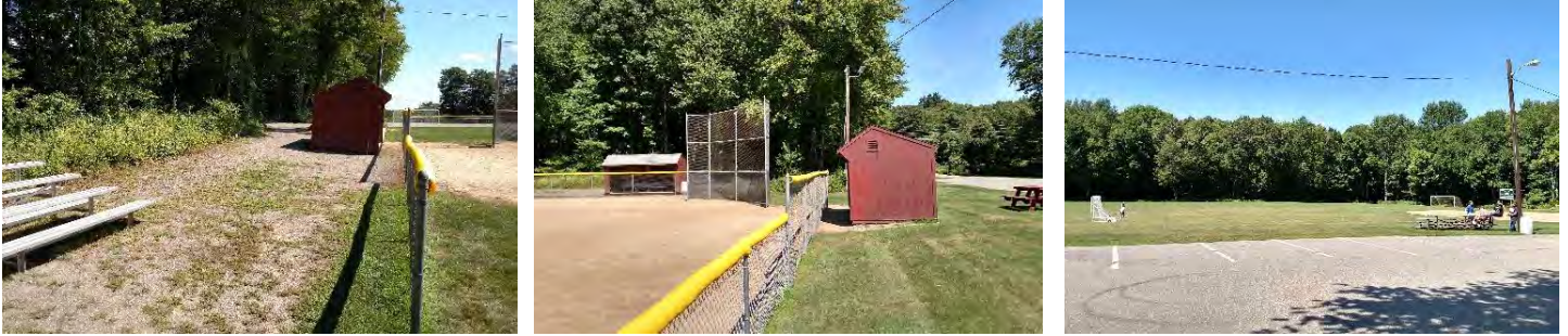
The image at left shows the area where there are drainage issues at the softball field. All images above also show the lack of accessible viewing areas at the field. The image at right indicated the overlapping nature of the field. Note, the little league baseball field has an outfield fence, creating a gender inequity at the softball field.
